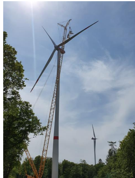
First Wind Works project built after the market crash in 2017, 16.5 MW wind farm Wald, Germany
