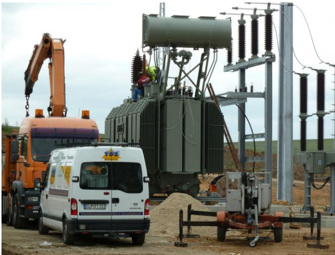
Wind Works 110kV Transmission Facility
